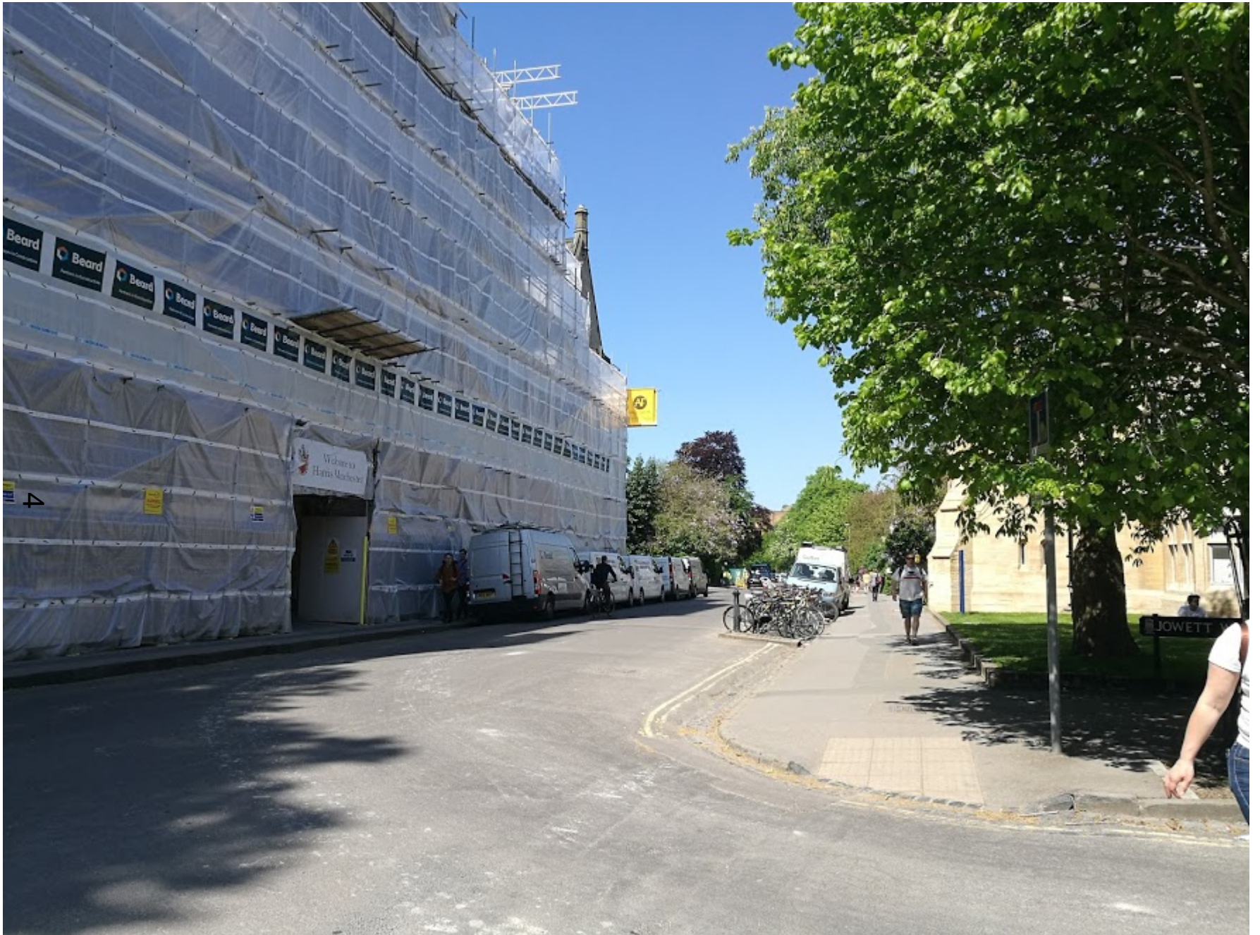
View of site from Junction of Mansfield Rd and Jowett Walk, Harris Manchester's library to LHS
